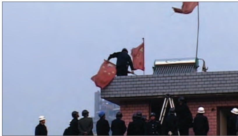
Picture 8: the Police removing flags the residents hoisted on the roof of their home before proceeding with demolition. This image is captured from a video film taken by one of the residents.
